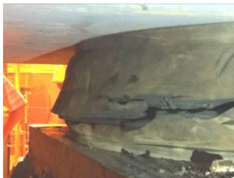
(a) Rubber bearing layer ruptured (S-3)
